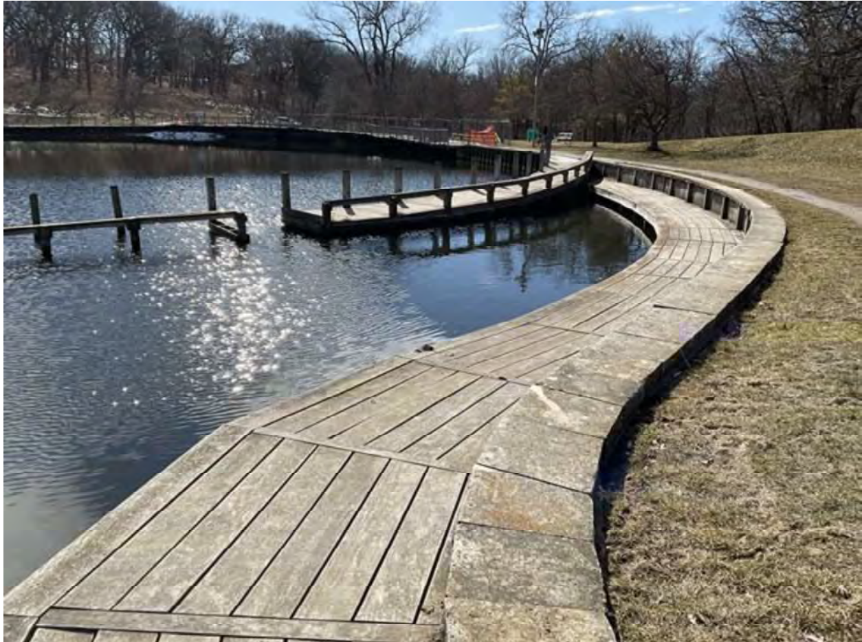
Inherent wear, warping, and decay of wood on walkway.
