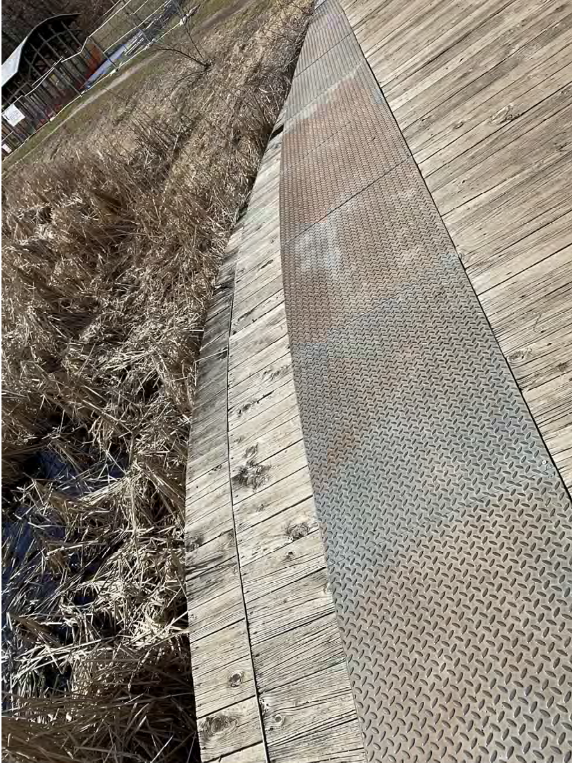
Wear, decay, and loss of wood elements on the bridge. Metal components rusting.
