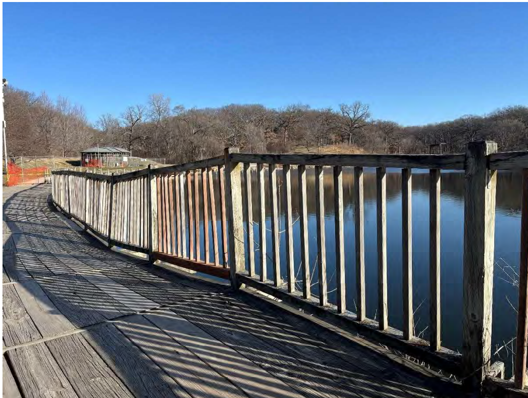
Figure 2. Condition of the boardwalk.
