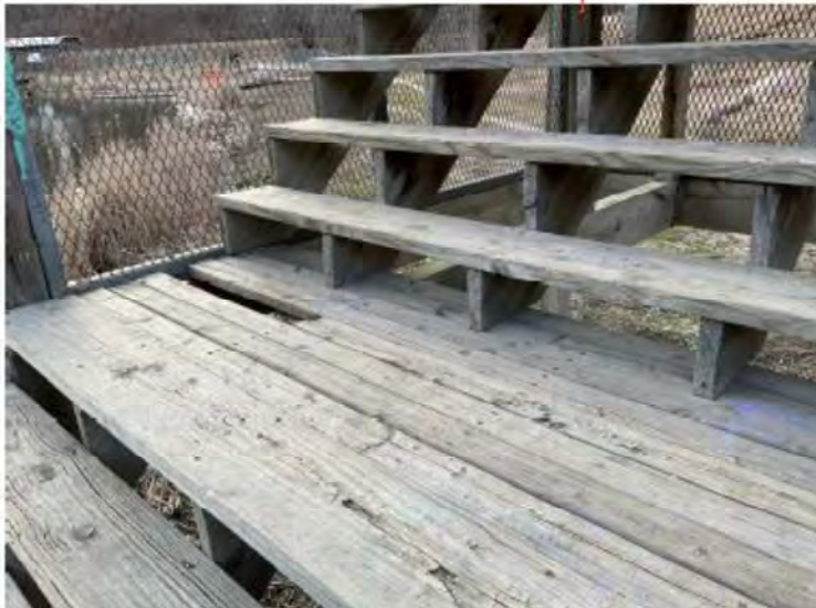
Detail of loss on first landing.
