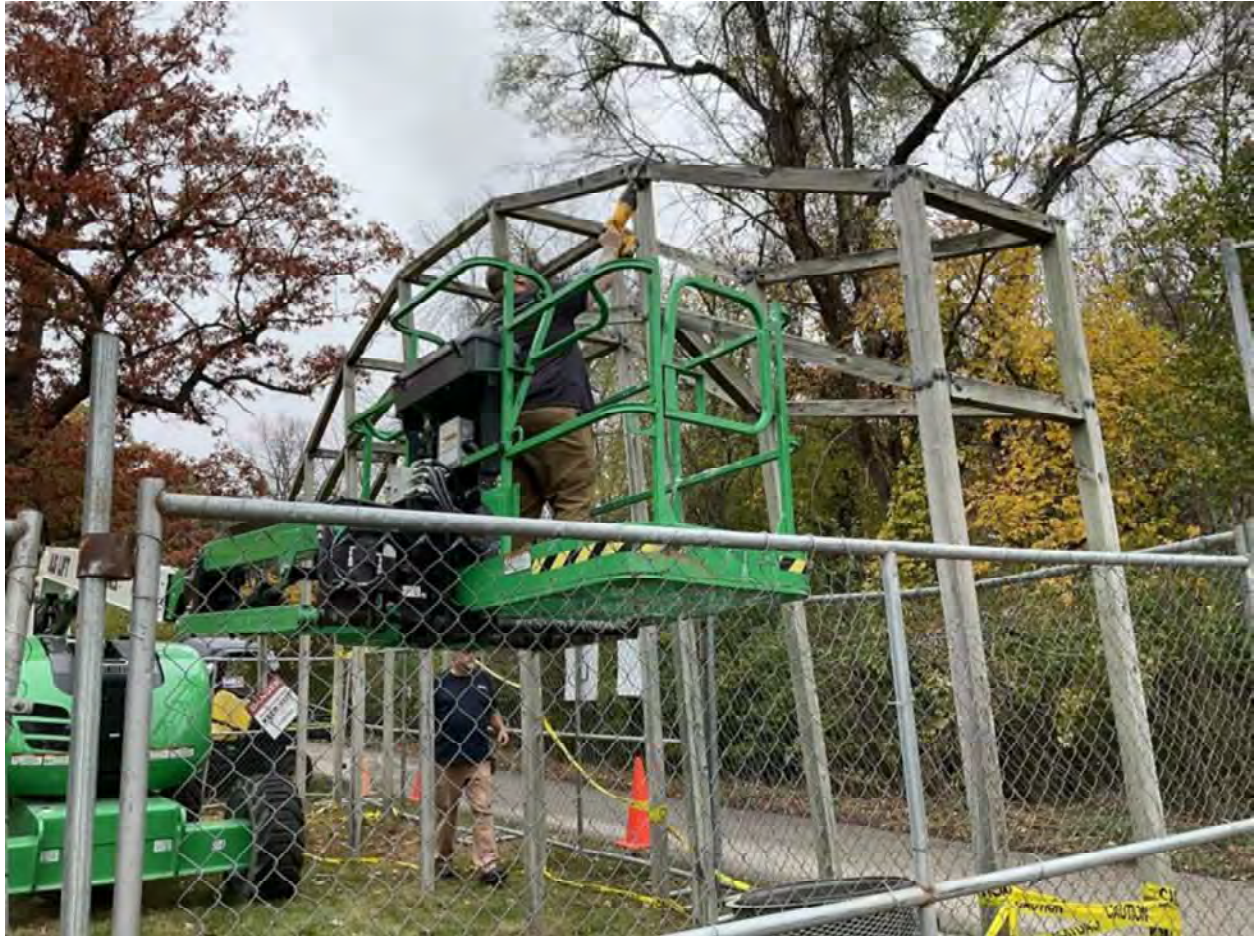
DMAC Director of Facilities and Lead Facilities Manager deinstalling the freestanding structures, October 2023.
