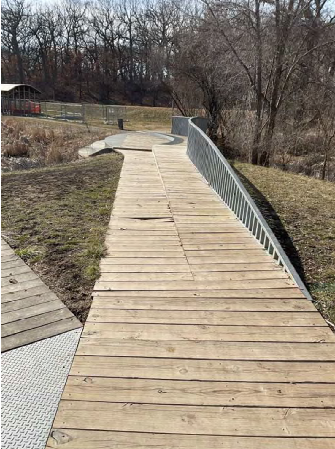
Visible warping, wear and decay, cracking, and losses of wood approaching the bridge.
