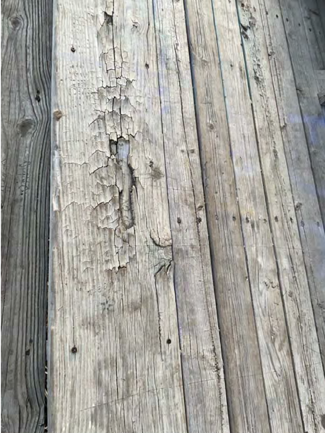
Detail of wood condition.
