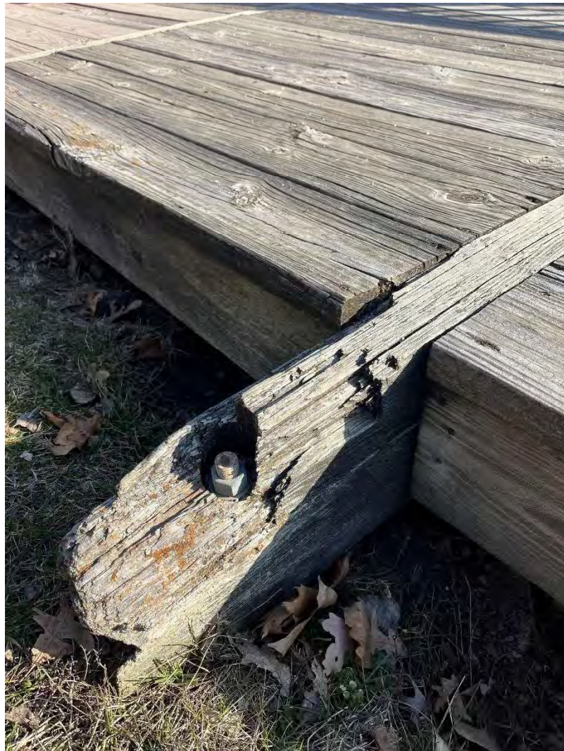
Figure 3. Condition of a boardwalk hold down.
