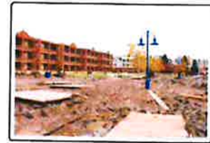
Damage to Duluth's lake walk Photo by Greg Johnson
